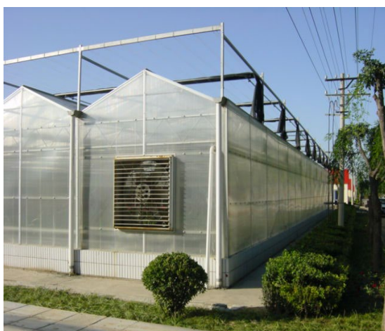
Pad/fan system and a movable outdoor screen
